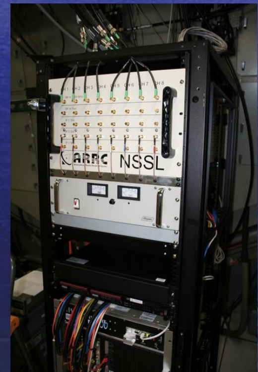
Installed rack w/ digital receivers
